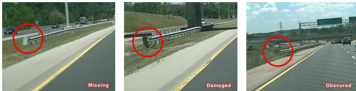
Figure 24: Examples of Missing, Damaged and Obscured Object Marker Signs
