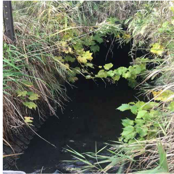
Photograph 26. ↑ WC-09. Water present at culvert outlet.
