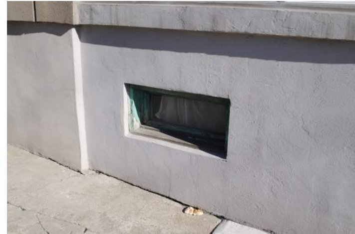
View of 81 Wilson Street, looking east towards the front porch. This small window frame, in poor condition, is likely an original.
