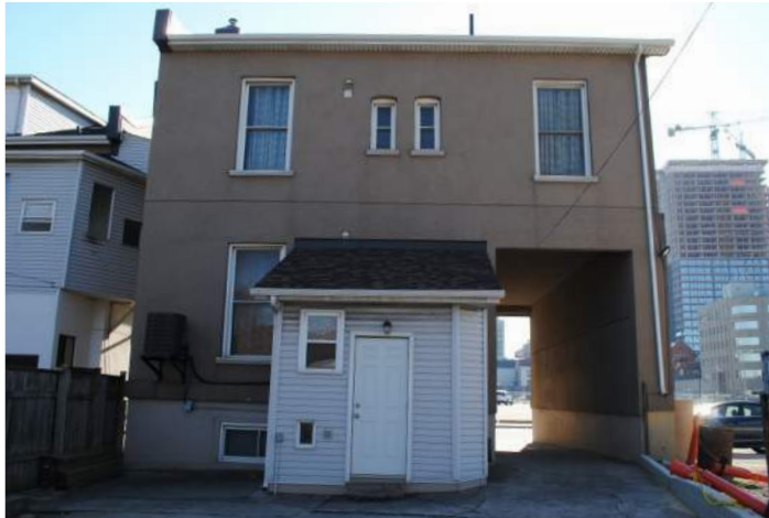
View of 81 Wilson Street, looking south from rear property. The Porte-cochère is visible at right. All evidence of original materials has been removed, and original brick has been re-clad with modern stucco, likely damaging the original face brick irreparably.
