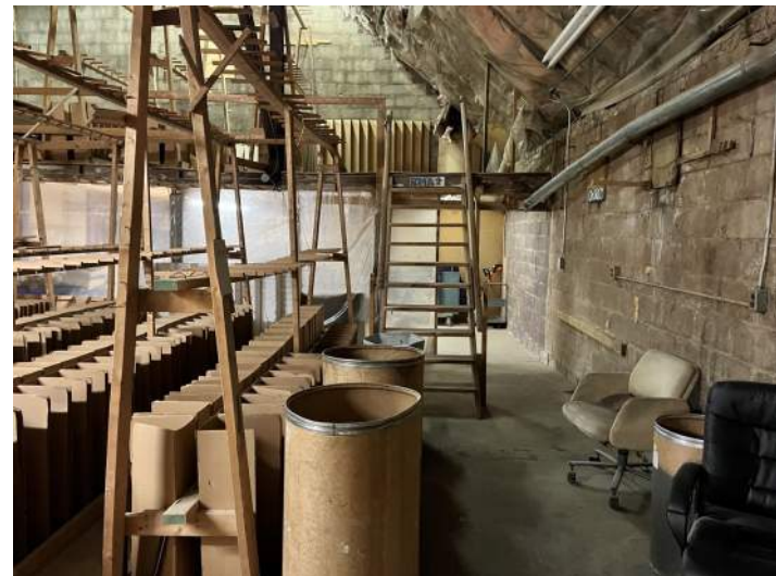
View unfinished first level work/storage space, looking east towards end of structure.
