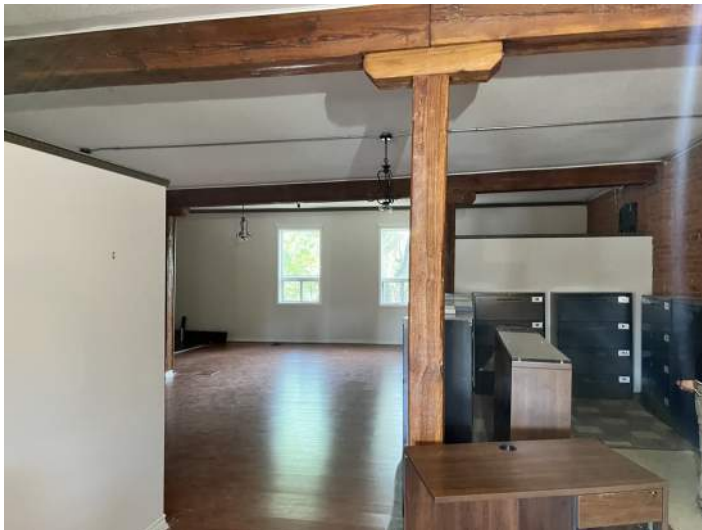
View second level modified commercial space at 100 John Street N, looking west. Original wood columns and beams are visible.
