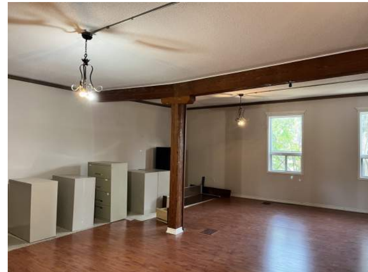
View second level modified commercial space at 100 John Street N, looking west. Original wood columns and beams are visible.
