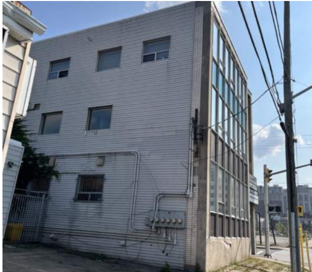
Looking south towards north elevation of The Gary Procter building. Aluminum siding has been applied to this elevation.
