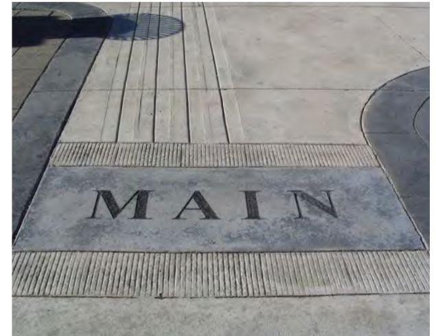
Accent areas, located outside of the pedestrian clearway can be of various materials (example on Bay Street).
