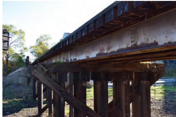
Plate 35: View of steel beam between timber supports and railway track looking south
