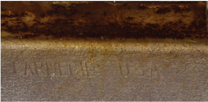
Plate 4: Carnegie USA inscription on west portion of steel beam on timber trestles
