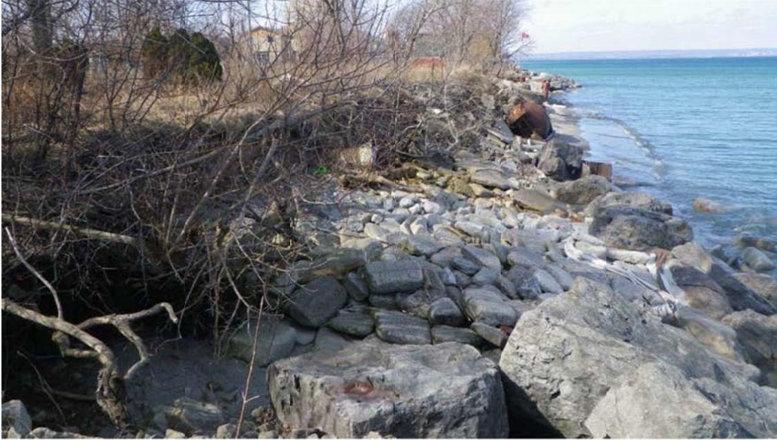
Figure 2.4: View of Rubble and Armour Stone in Central Part of Site, Looking West
