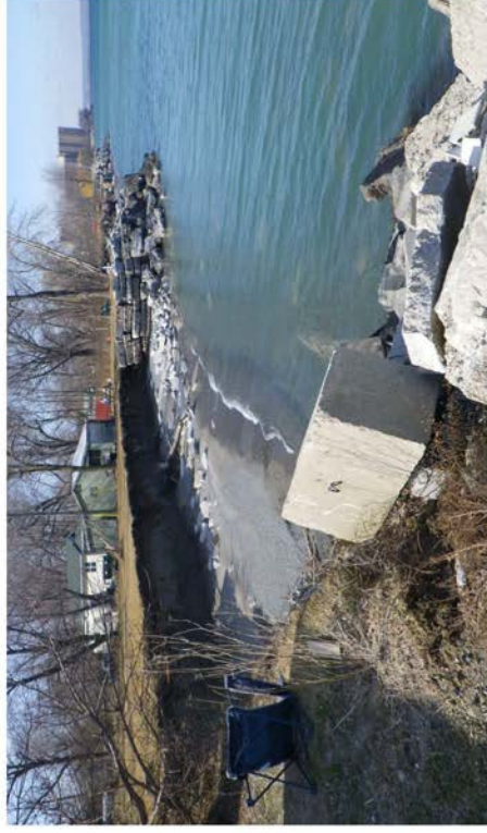
View of Eroding Bank in Eastern Part of Site, Looking West
