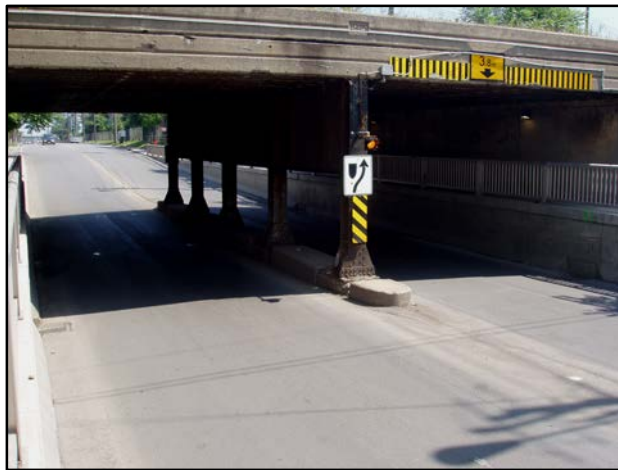
Recurrent flooding at the Kenilworth Street Bridge. July, 2006. Photo credit: City of Hamilton.
