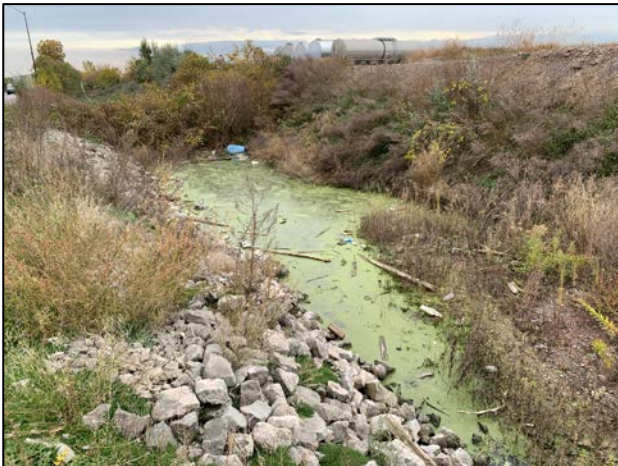
Middle portion of Eastport Ditch 3 showing bermed area at end of growing season. Facing south
