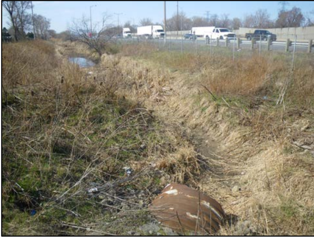
Upstream end of CSP pipe connecting downstream end of Eastport Ditch 2 to Eastport Ditch 1, facing upstream (NW)
