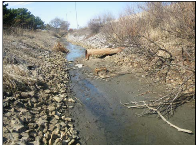
Eroded storm water outlet pipe midway upstream in ditch, facing NW. Note sediment accumulation
