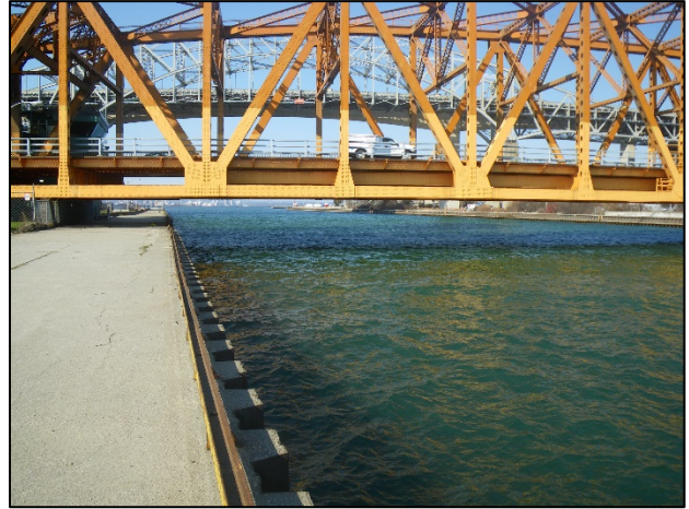
Central portion of the Burlington Canal facing west. Note lift bridge (Eastport Drive) in foreground and Burlington Skyway (QEW) in background
