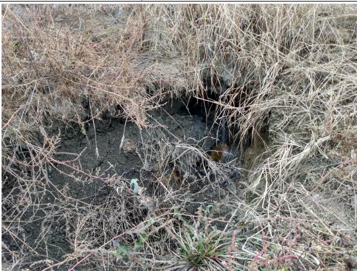
Headcut formed where surfaced water flows down into broken tile drain. Downstream of this headcut, baseflow is conveyed subsurface through the tile drain.
