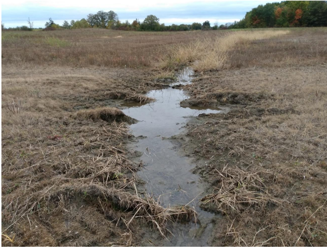
Upstream view from culvert. Watercourse banks appear to have been impacted by crossing of agricultural machinery.
