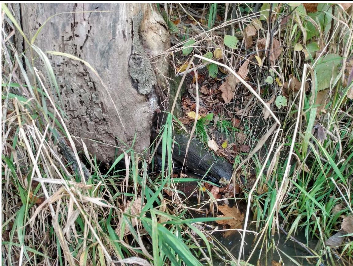
Exposed tree root along outer bend of channel near downstream extent, indicating minimal local erosion.
