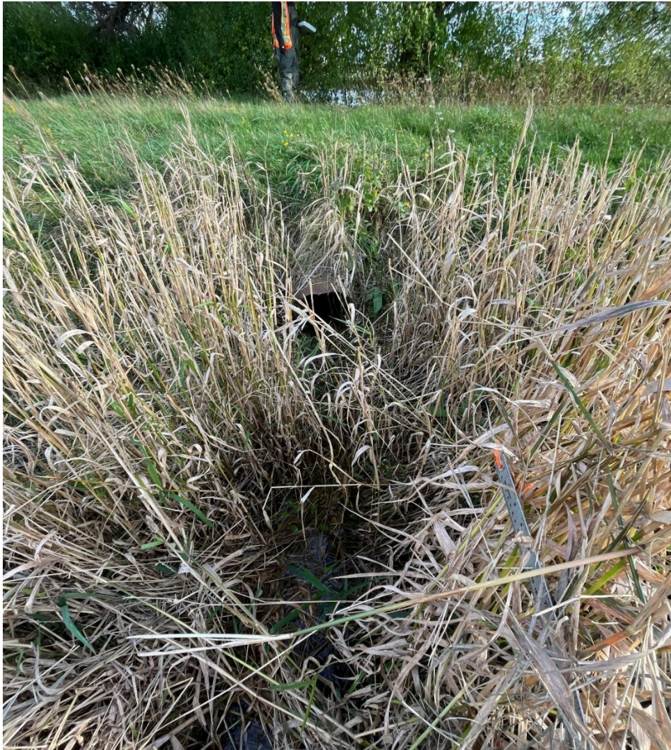
Photo 43: 3-SC1 Pond (October 23, 2025). Tile drain outlet connecting to pond.
