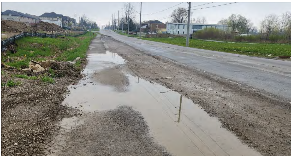
Figure 2.1) West 5 th Street Sidewalk Condition – Drainage
