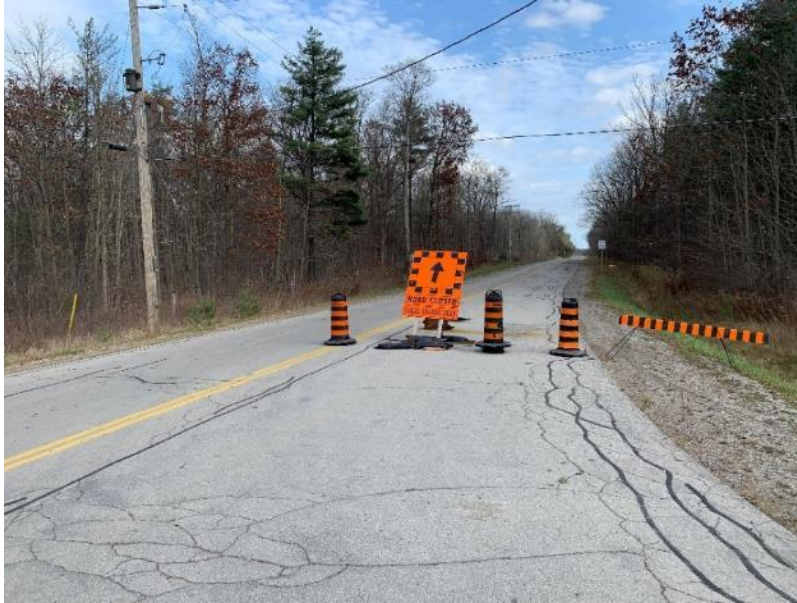
Image 1: Safari Road closure warning sign due to localized flooding. Test pit survey required beyond disturbed, elevated roadbed.
